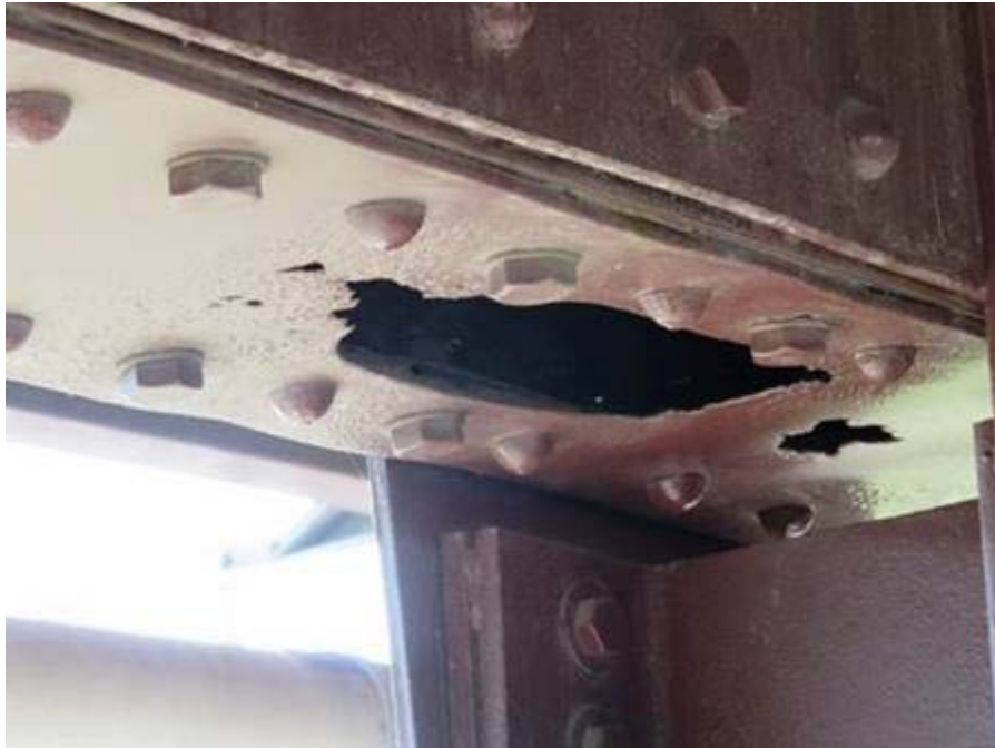
Str. 6416 – photo 1: Corrosion holes in bottom face of member U16-U15WB near U16WB
